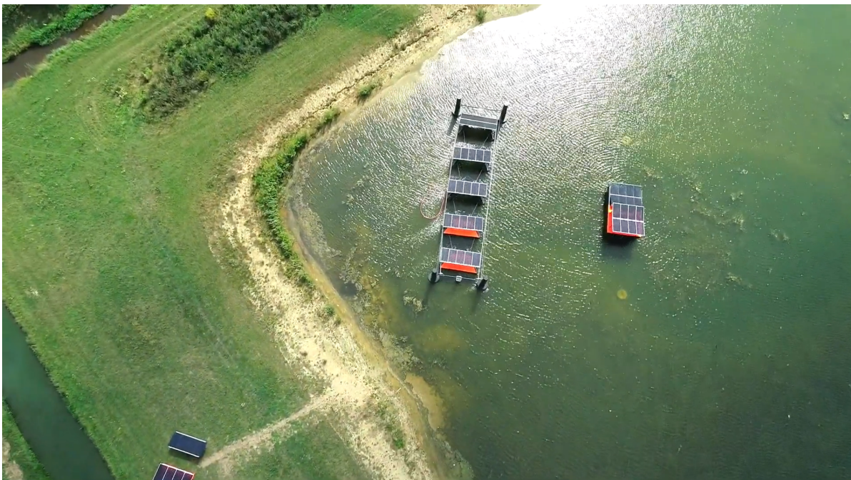
Figure D.1: Bird's-eye view of the INNOZOWA PV Pilot system. Adapted from: https://www.youtube.com/watch?v=wZT82wG19ck .
