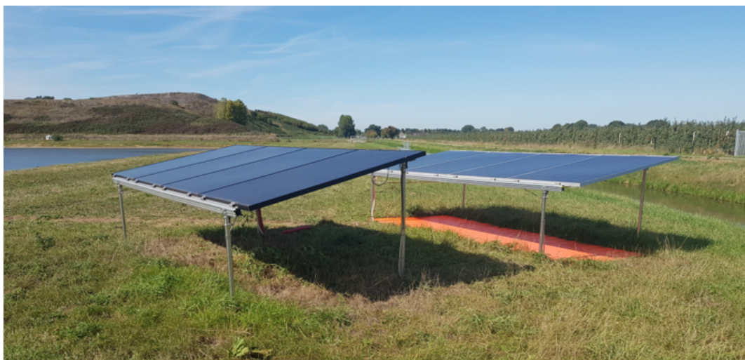
Figure 3.1: On-site photograph of the Ground-based System, installed for the INNOZOWA pilot project.
