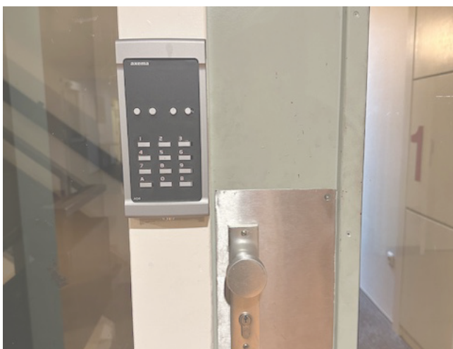
Image 39: Lock on an exit (Own work, 2024)
