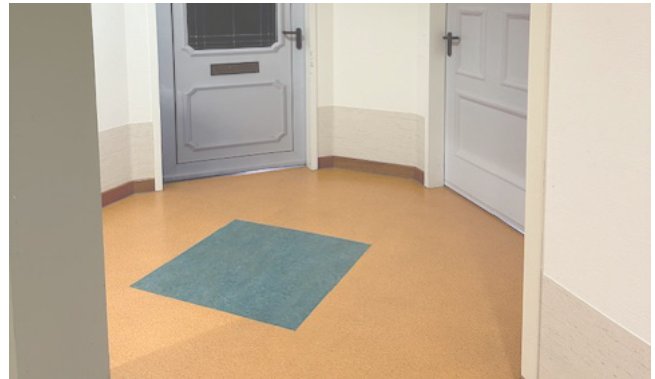
Image 20: Green patch on the floor (Own work, 2024)
