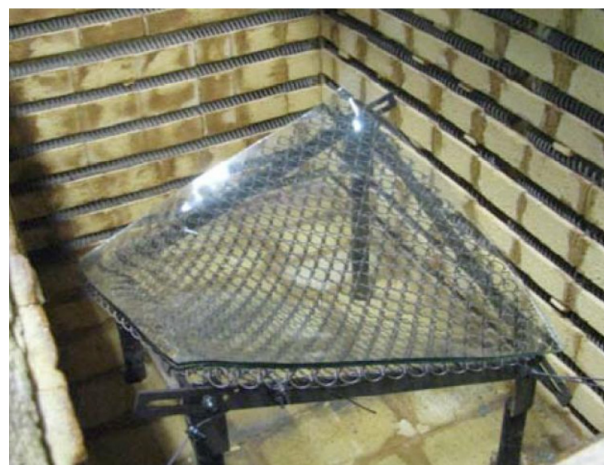
Figure 64: ‘Sierra Papa 2’ before and after hot bending of glass. Source: Schuurmans & Pronk, 2011.
