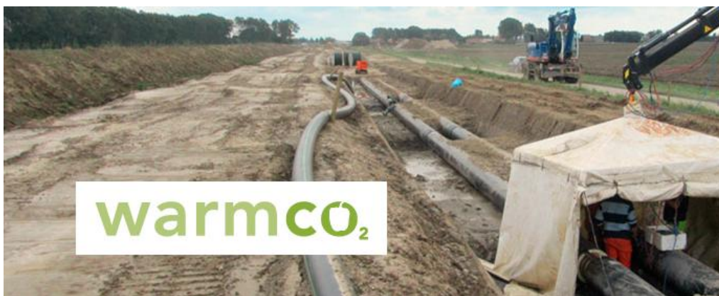
Figure 11 – laying of the pipelines needed for the exchanges managed by WarmCO 2 (Source: www.warmco.nl )
