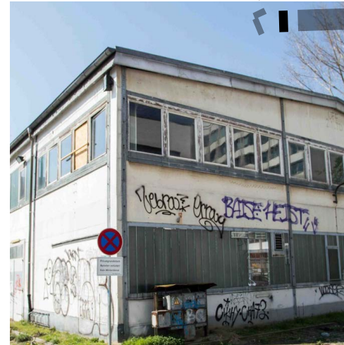
BADLY AGED FACADES
