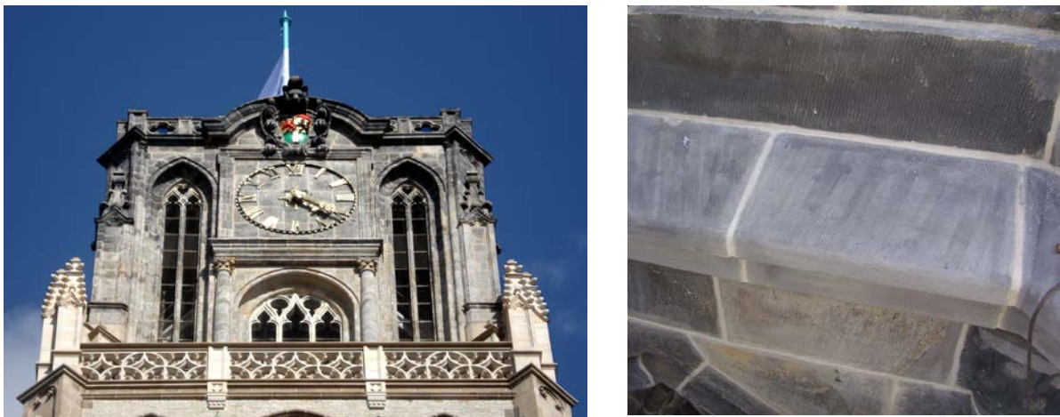
Figure 3 Application of an artificial patina on new sandstone to visually match old sandstone at St. Lawrence Church Rotterdam (photo left: W.J. Quist, photo right: T.G. Nijland)
