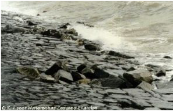
Figure FS5.4: Damage to a pitched basalt revetment
