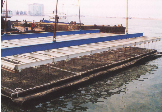
Figure FS7.1: Placement of a large open stone asphalt mattress with a lifting frame (Bitumarin)
