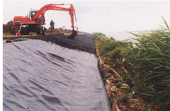
Figure FS7.2: In-situ installation of open stone asphalt with a crane (Eemmeer)
