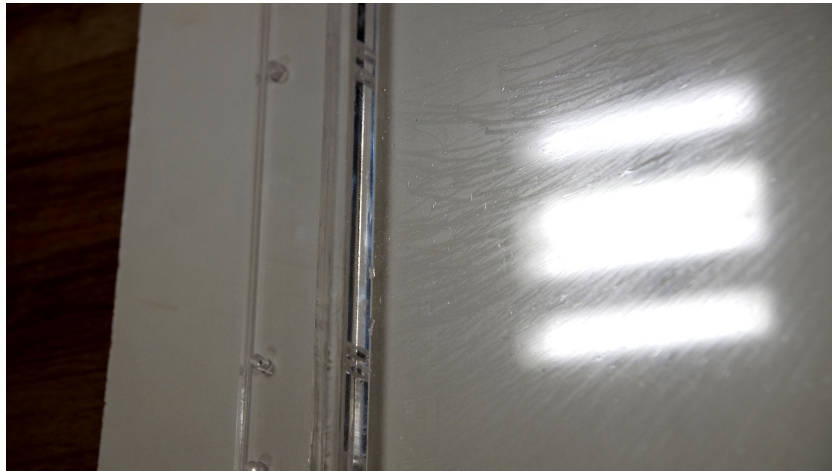
Figure 4.11: Streaks of DEHS oil that has settled down on the inside of the channel. Picture shows part of a door that was removed at the time.
