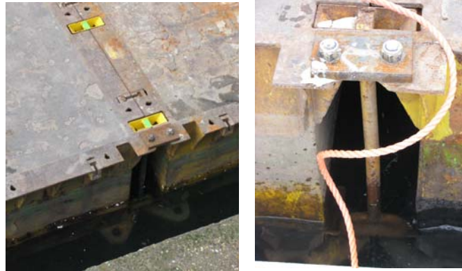
Figure 22: Connection pontoons Heijsehaven, vertical element with double pen below, securing bolts above
