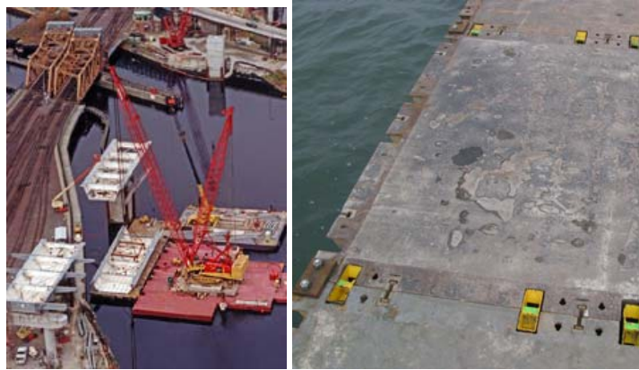
Figure 8: Left, Steel Flexifloat pontoons with crane on top (Flexifloat) Right: picture pontoons Heijhaven.
