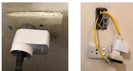
Fig. 2. Plug-wise unit installed for energy measurement
