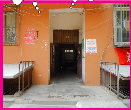
POORLY MAINTAINED INFRASTRUCTURE
