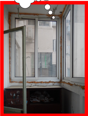
POOR CONSTRUCTION QUALITY
