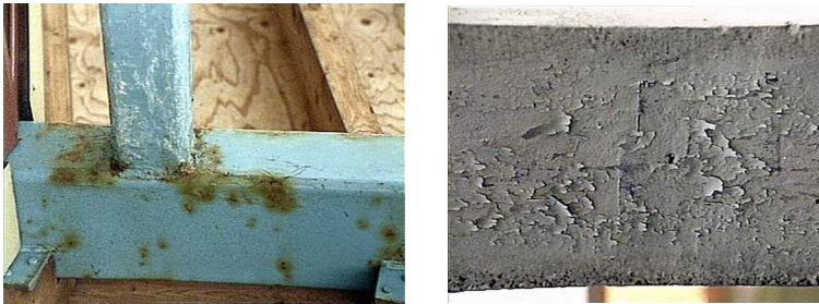
Fig. 2 Photo's of coating degradation. Left: coating degradation leading to corrosion. Right: coating degradation leading to flaking of coating.
