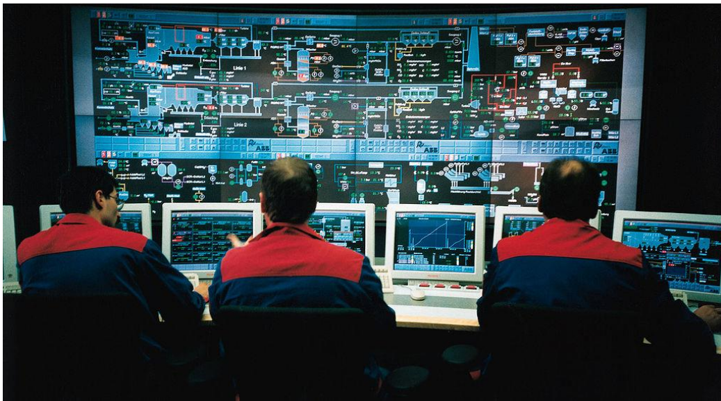
Figure 3. A photo of SCADA system 2 .
