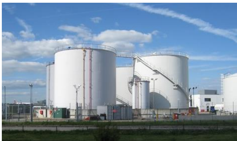
Figure 44. An example of typical storage tanks
