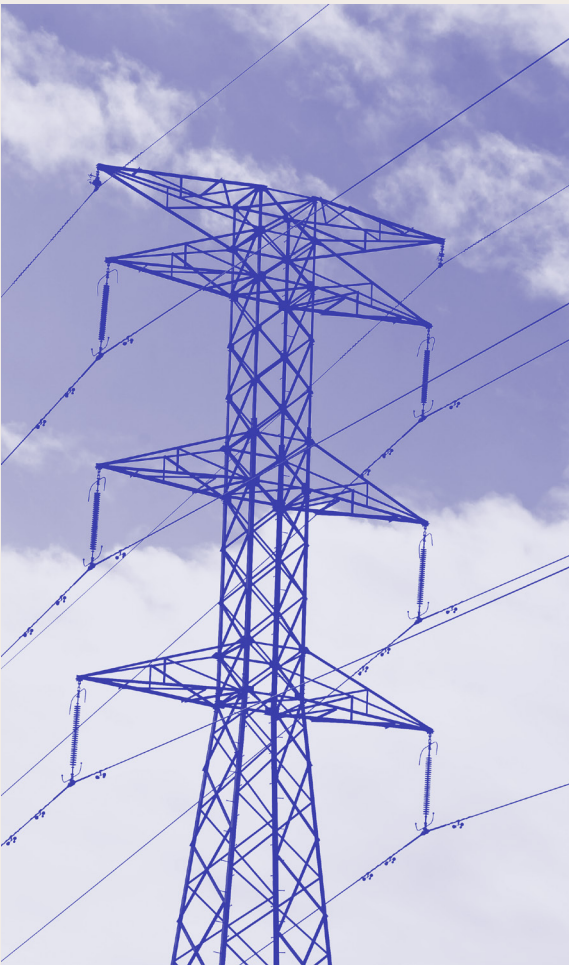
Figure A.6: High voltage pylon Source: Freepik
