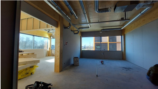
(b) Picture: floor plane axis A-B where the architectural finishing and installations are visible
