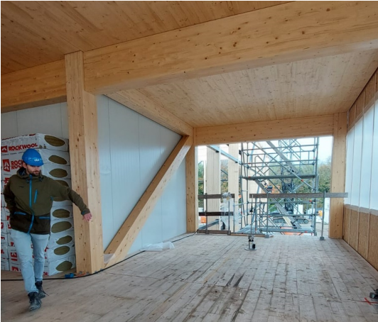
(a) Picture: floor plane axis F-E where the structural timber is visible
