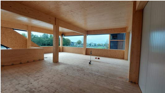
(b) Picture: floor plane axis A-B where the structural timber is visible
