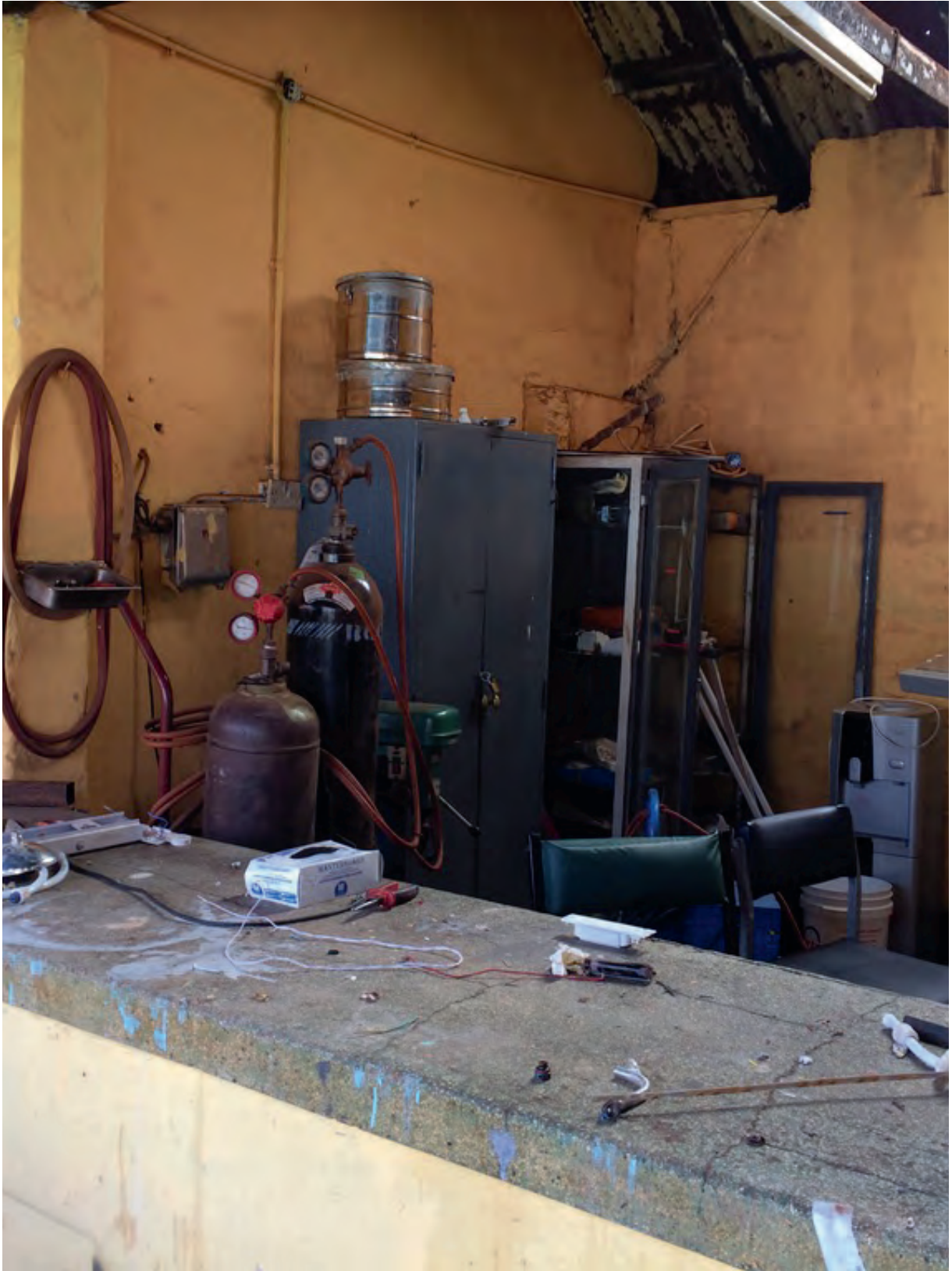
Biomedical engineering equipment technicians workplace in a large hospital in Kenya.
