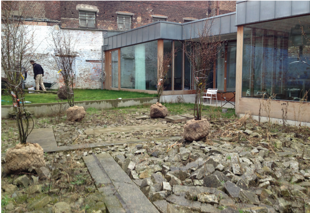
FIGURE 3 Construction of a framework for the different garden zones through differentiated soil treatments. The design of the central garden (bottom half of the picture) literally breaks through the sealed character of the site by scattering the concrete slab into the plant substrate. Several strips of concrete are left unscattered to be used as pathways. The plantings of Amelanchier ovalis ensured the client of the direct presence of structuring green. In the upper garden (top half of the picture), reachable by a concrete step, the concrete slab was fully removed and grass with two Celtis occidentalis was provided. This approach enabled different modalities of floral and human recolonisation and in doing so stimulated a variety of garden experiences. (Photograph by Geert Meysmans, 2013. Reprinted with permission).
