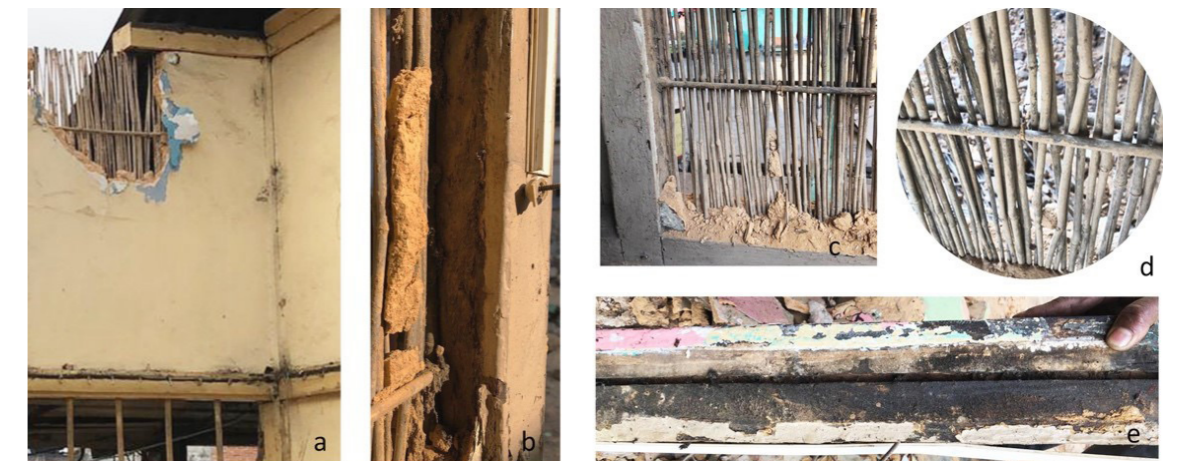
Figure 7.28: a) Connection of the Ikra panel to the wooden columns, b) The plaster sticks on the rough surface of bamboo, c) The central tie that runs through the vertical bamboo sticks is inserted into a hole in the wooden member, letting it free to move, d) metal wire or bamboo threads are used to ties the horizontal members of the bamboo together, e) a groove is cut on the horizontal wooden members which run above and below the thin bamboo sticks, the sticks slide into this groove which acts like a channel. The wooden member is then connected to the vertical posts.
