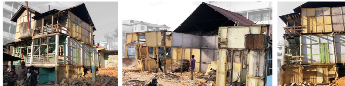
Figure 7.23: Images of the measured Assam-type construction on site, dismantling of the construction was in process.
