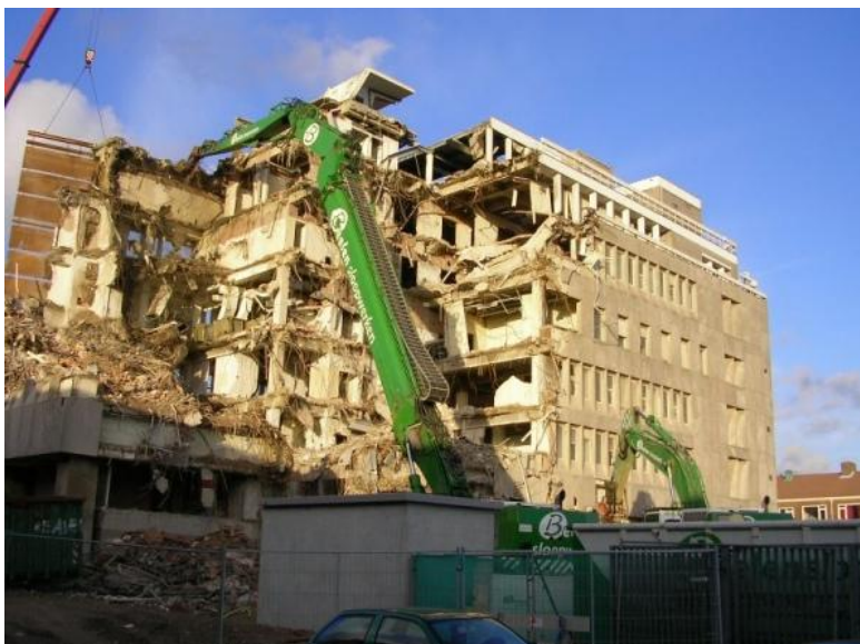
Figure 2.19 - Low rise demolition of the PCH operational building in Ijmuiden with an excavator [Source: coastradio.intco.biz/]
