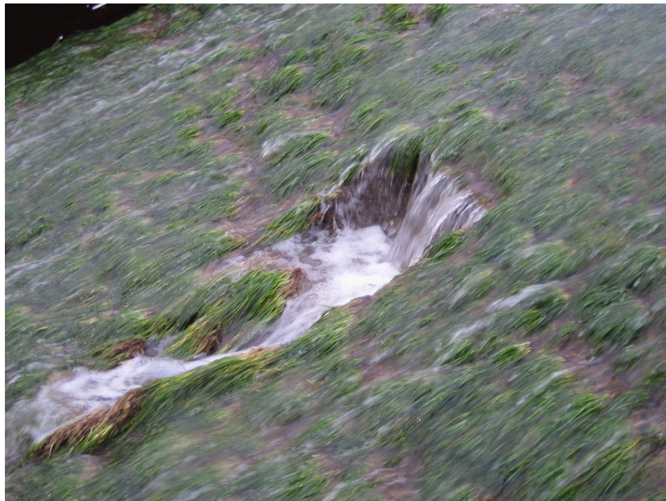
Figure 18: Flow concentration in the locally damaged grass revetment
