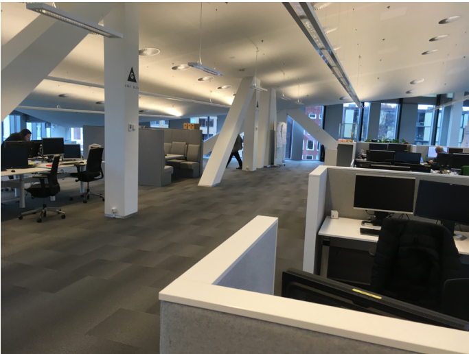
Figure 5.1: The crooked beams can seriously injure employees.
