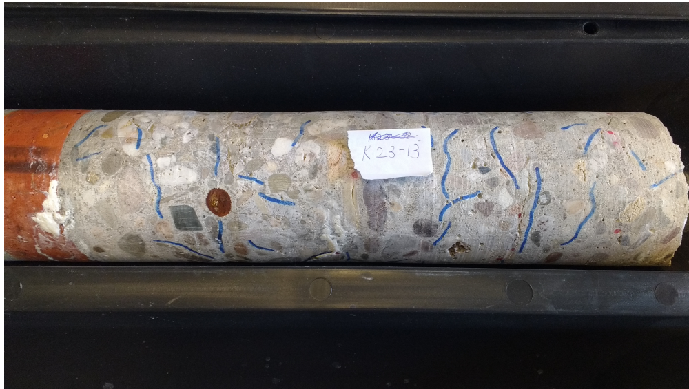
FIGURE 3.6: Example of a concrete core. Tag Number K23-13. The micro-cracks observed in the visual expansion are marked in blue. The left hand side surface indicates the brick masonry layer on the top.
