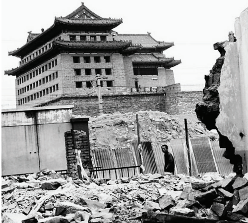
Figure 3.2: Demolition for creating 'available land' for new development (photo by Getty Image)
