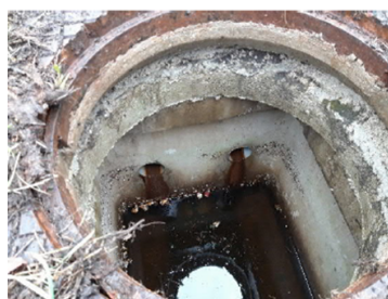
Figure 3.9: In the blue trajectory the drainage pipes are located above the stormwater conduit (below water level in picture) (Zwart, 2020).
