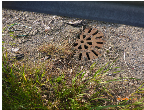
Figure 7.1: Dirty open manhole near 119.0 (Van Den Biggelaar, 2021).
