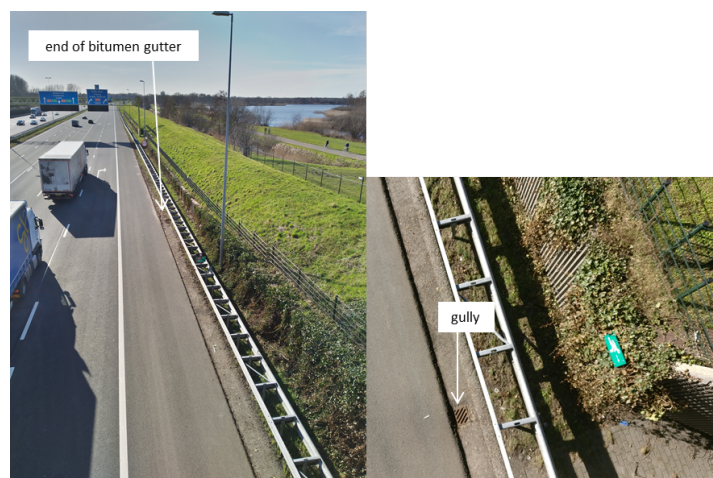
Figure 3.11: Bitumen gutter with rectangular gutter in northern verge near junction Sint-Michielsgestel (Field visit 24-02-2021).
