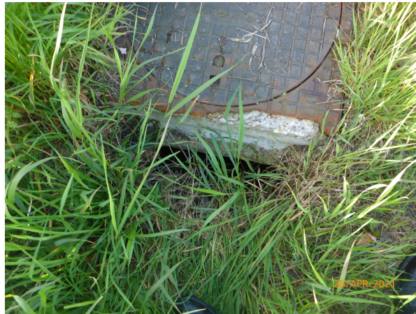
Figure 8.1: Wash-out of the soil near a closed manhole near 119.1 (Van Den Biggelaar, 2021).
