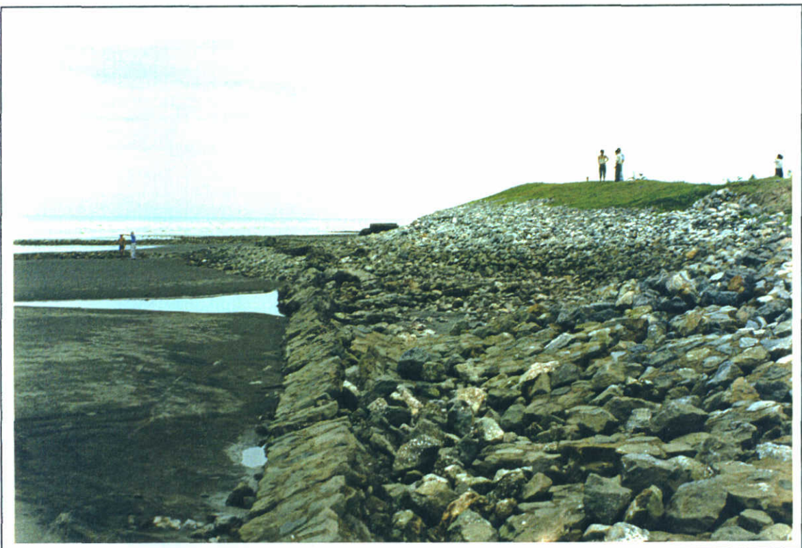
Photo 6 Cement enforced toe, groins and slope protection damage
