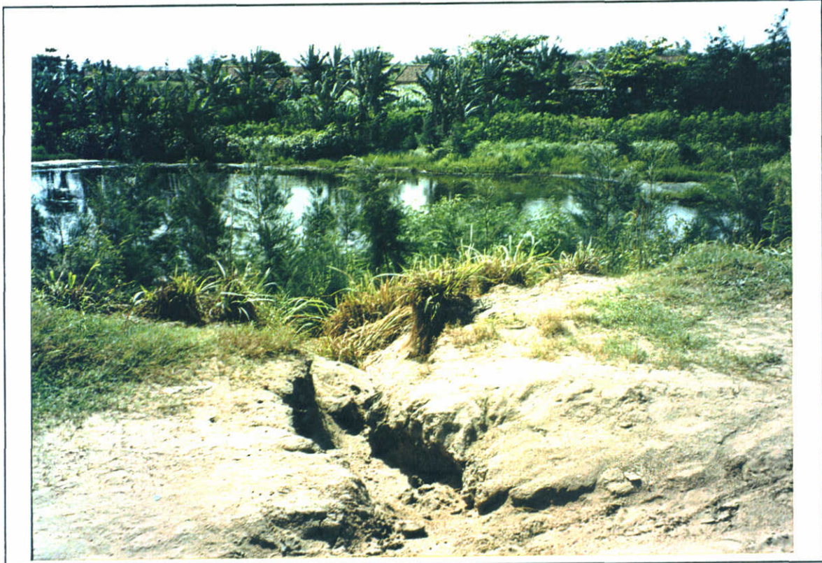
Photo 9 Backside crest erosion due to overtopping near Hai Thrieu
