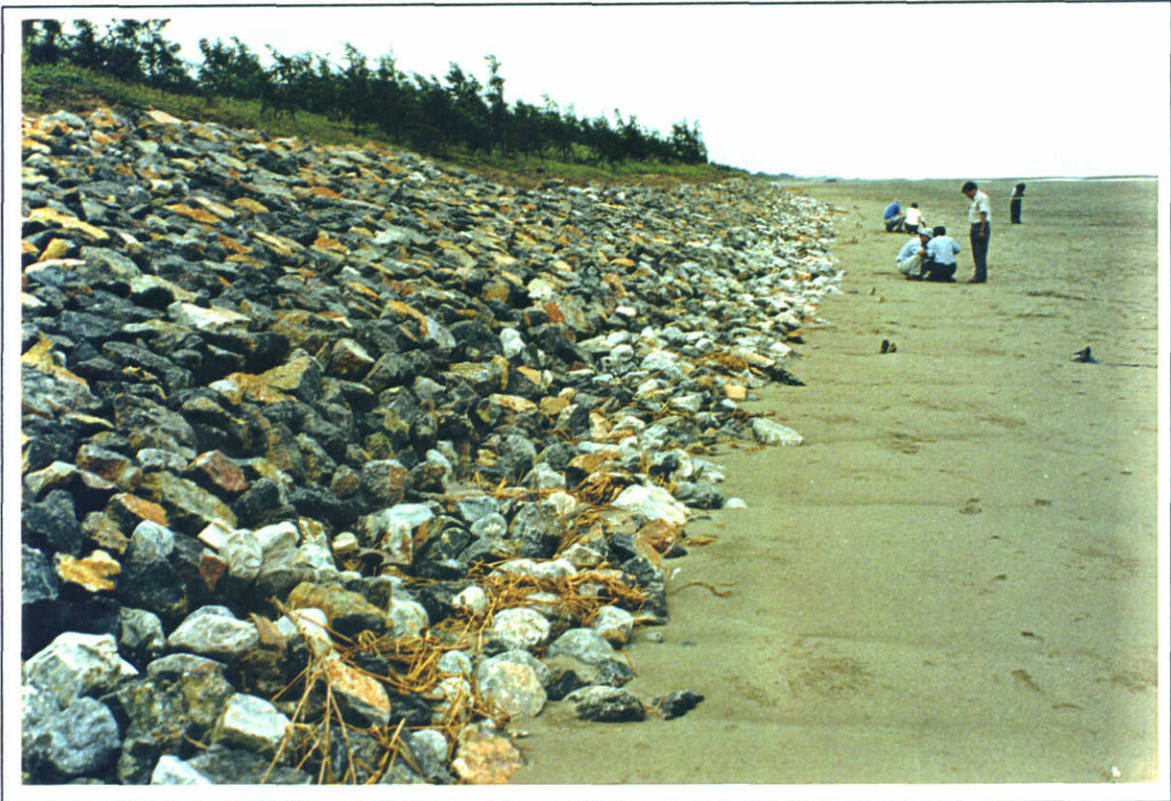
Photo 5 Slope protection, exposed toe
