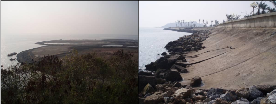
Figure 18: Construction of artificial islands in Do Son (left) and state of the sea wall (right) [photo: Hillen]
