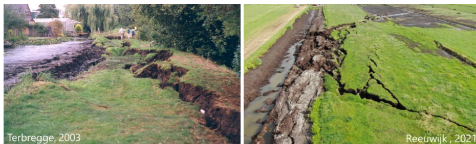
Figure E 1 Left: The dike breach at Terbregge, The Netherlands, in 2003. Right: the dike breach at Reeuwijk, The Netherlands, in 2021. In both cases, the canal is on the left side and the polder is on the right side. The canals were rather shallow and up to about one meter deep, limiting the development of the breach and the water that could flow into the polder.
