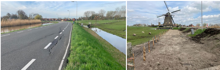
Figure 6.2 Settlement and crack formation along the regional flood defences near the N468 between Schipluiden and Maasland (left). The ditch next to the dike has been filled with sand to reinforce the dike (right). Pictures from the water authority of Delfland.
