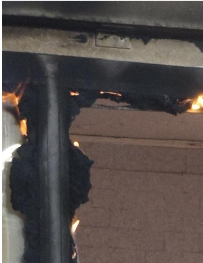
Figure 2.16 Too much intumescent tape in Test 1 (failed)
