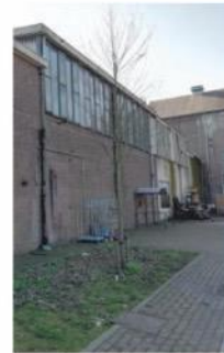
407-unusable due to the extent of decay
