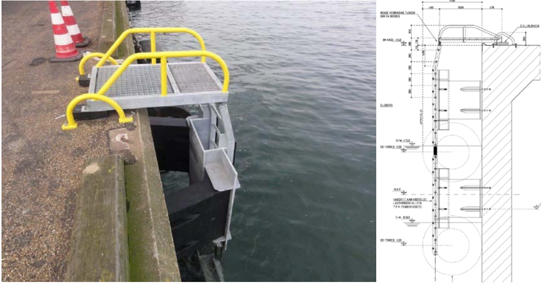
Figure 9: barge ladder between cylindrical fenders to provide barge access (photo PoR)
