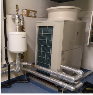
(a) Air-to-water HP.
