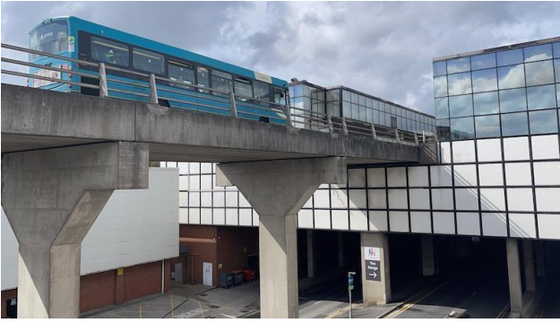
FIGURE 3.12: ELEVATED PART OF THE RUNCORN BUSWAY GOING INTO THE SHOPPING CENTRE (FRENCH, 2022).
