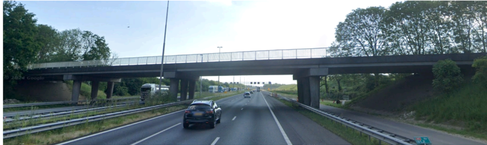
b) View of the Ardeweg viaduct from the A1 motorway, facing north [49].
