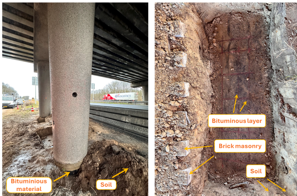
Fig. 5. Exposure environments of structural members: (left) columns partially coated with bituminous layer at the lower section of their height and surrounded by soil and brick masonry; (right) foundations coated with a bituminous layer, in direct contact with soil and brick masonry.
