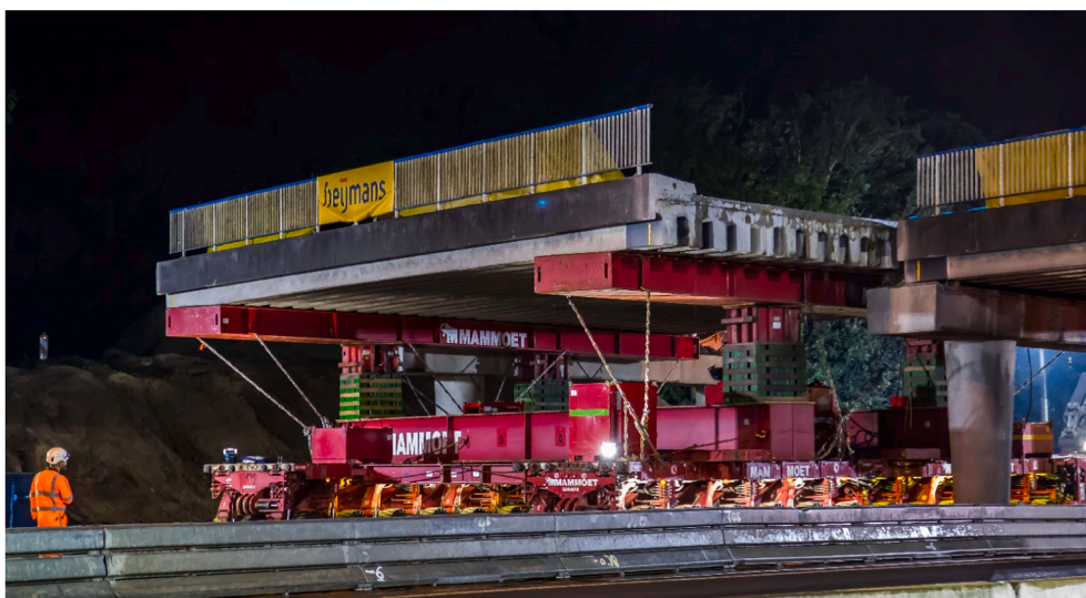
d) The deck 2 is gradually being dismantled and removed to the designated drop-off location [48].
