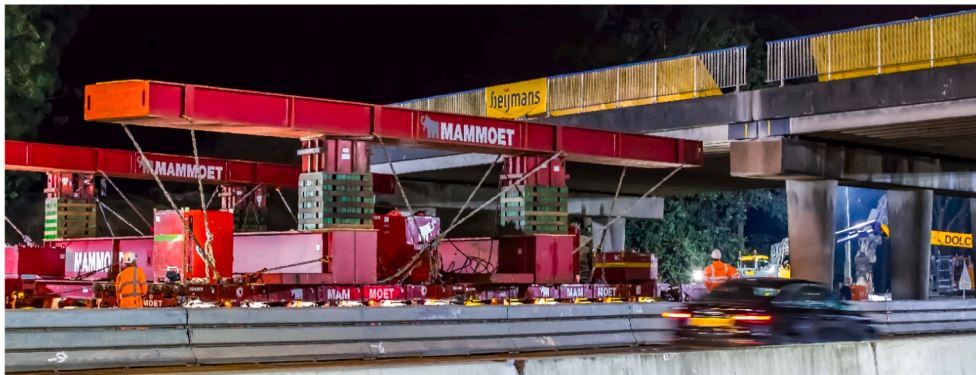
c) SPMT is positioned under the deck 2 to support and enable controlled movement of the structure [48].
