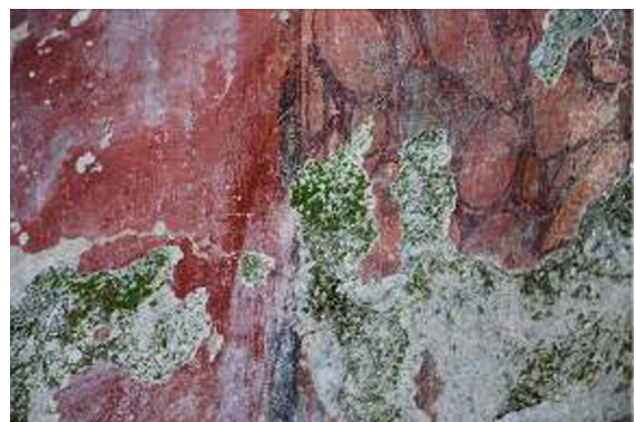
Fig. 8 Detachment and loss of a lime-based plaster from the masonry support. Archaeological site of Dion, Greece (Roman period): Plaster consisted of two layers of a total thickness of 2.5 cm (external: 0.5 cm, internal: 2 cm), decorated with wall paintings. (Photo archive: Lab. of Building Materials AUTH)
