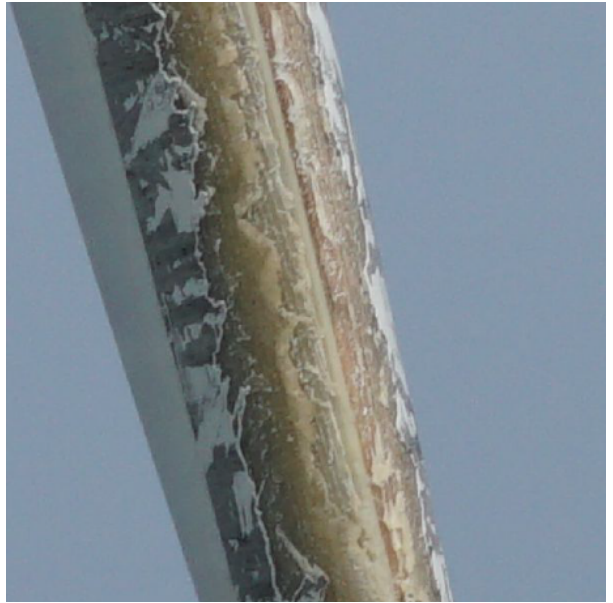
Figure C.21: Inspection April 2021, turbine 2, blade 3.
