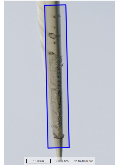
Figure C.19: Inspection November 2017, turbine 2, blade 3.
