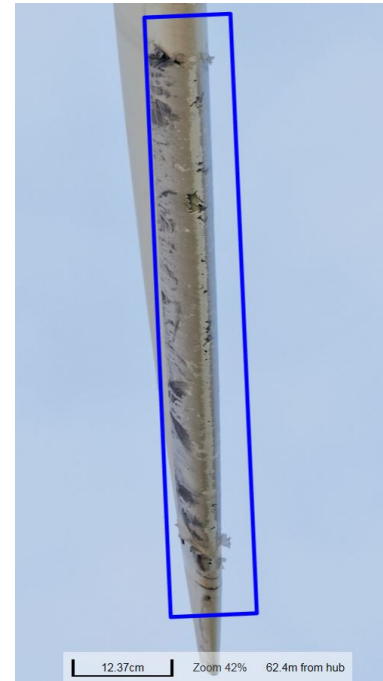
Figure C.35: Inspection November 2017, turbine 3, blade 3.
