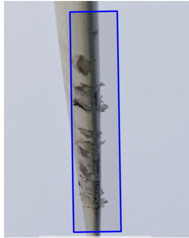
Figure C.18: Inspection November 2017, turbine 2, blade 2.
