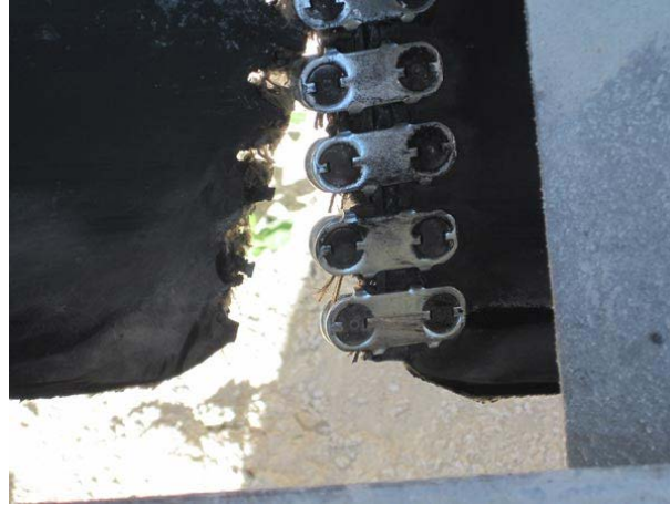
Figure 3.3: Belt breaking at the splicing area. Courtesy of BMG (2016).
