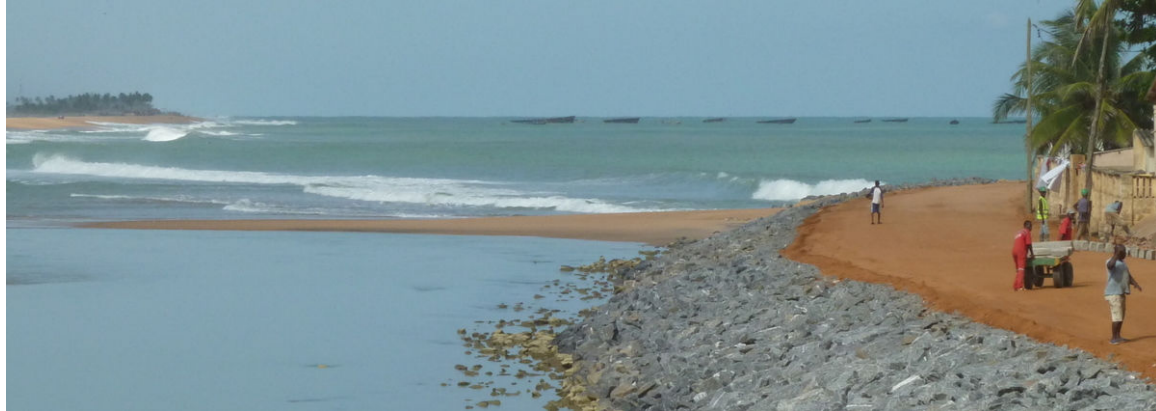
Figure 47 Revetments at Aného, west of the inlet. Continued erosion threatened the village of Aného.
