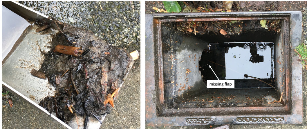
Figure 6-1 left: bed sediment from the gully pot with missing flap; right: gully pot without flap.
