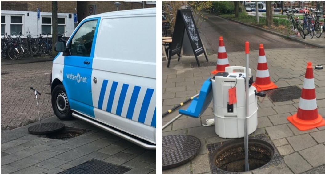
Figure D-3 Blocking of the road to take samples following the Waternet safety protocols.
