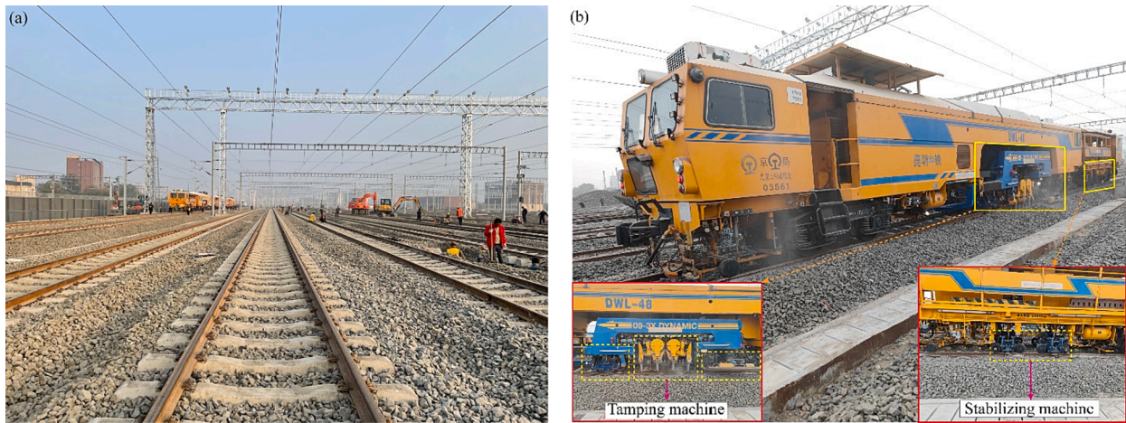
Fig. 1. Test site and tamping and stabilizing machines: (a) test site, (b) DWL-48 tamping and stabilizing machine.
