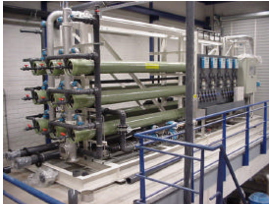
Figure 5. The Rodenmors nanofiltration plant (Vitens).
