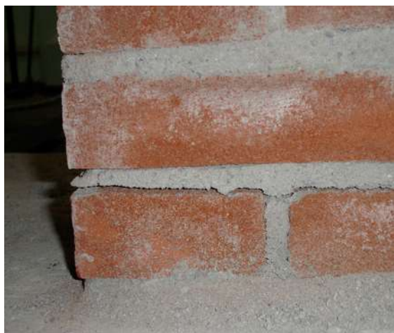
Figure 5.1: Tensile failure in masonry arch
