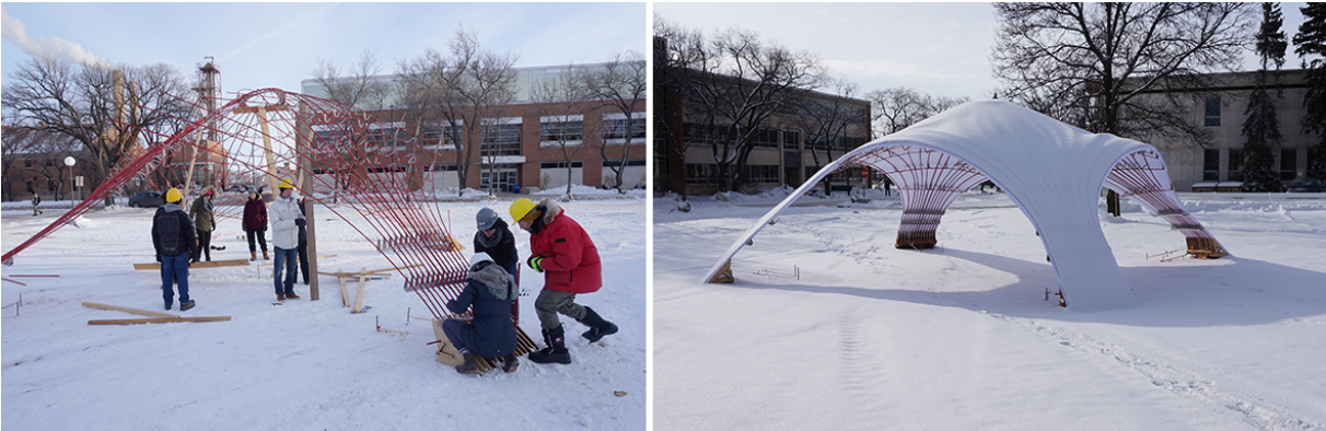
Figure 1: Students assembling the bending active framed vault (left), completed ice shell structure (right). [photos by Dominique Rey & Lancelot Coar]
