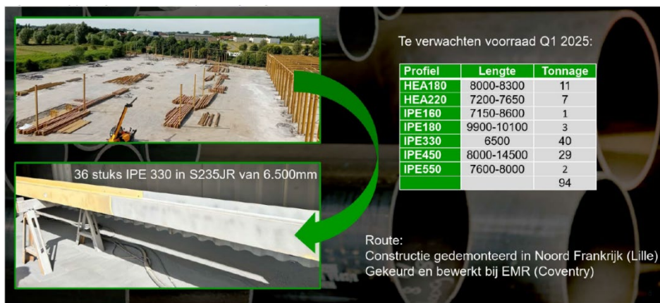
Figure 4.4: Construction stock demounted in northern France, tested and adapted by EMR (De Kok Staalbouw, 2023).
