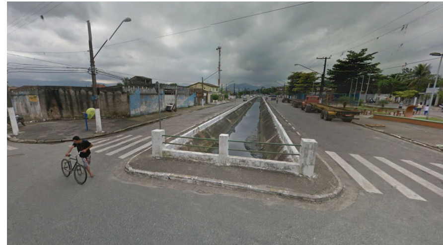
A canal on Av. Hugo Maia close to Vila Gilda. Due to a lack of capacity, it frequently floods. source: Google Streetview
