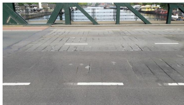
Figure 14 A wooden bridge deck fastens the deterioration process for wear layers
