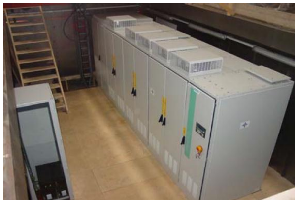
Figure 5-1 Flex Power Grid Lab: The converter
