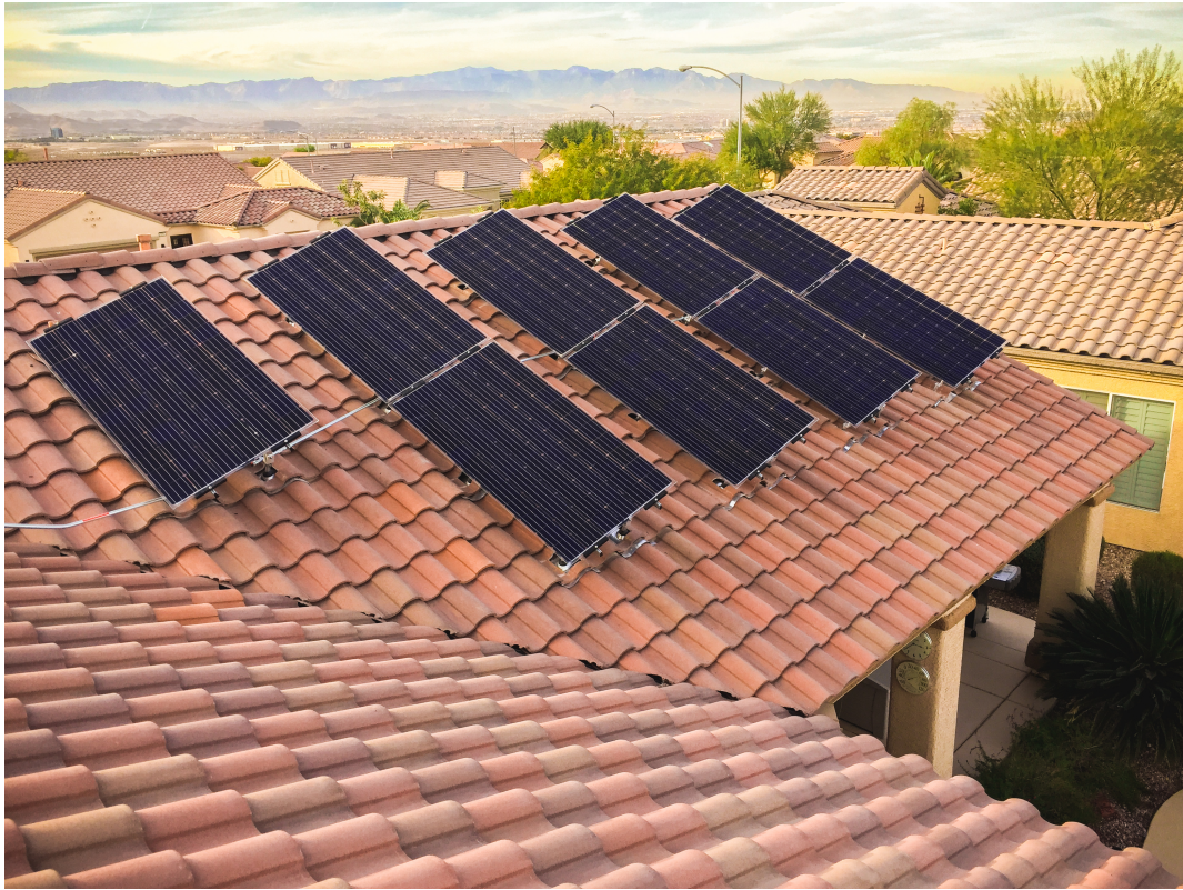
FIGURE 2.1: Example of a bifacial PV installation on a roof [4]
