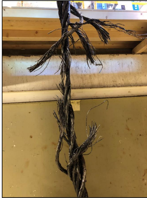
Figure 24 – Failure of the cable
