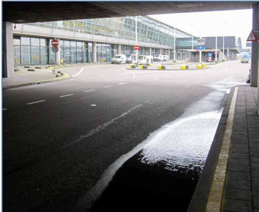
Figure 7.14; Beginning of the F-pier, no good drainage (07-11-2012, 13:11:01 PM)
