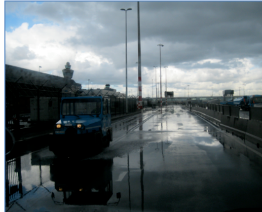
Figure 7.15; Photo of the RH-road (main axis) after rainfall (19-09-2012, 5:27:23 PM)
