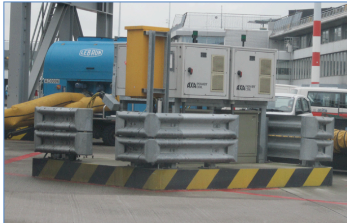
Figure 2.16; Ground Power Unit (GPU), fixed on large aircraft stands
