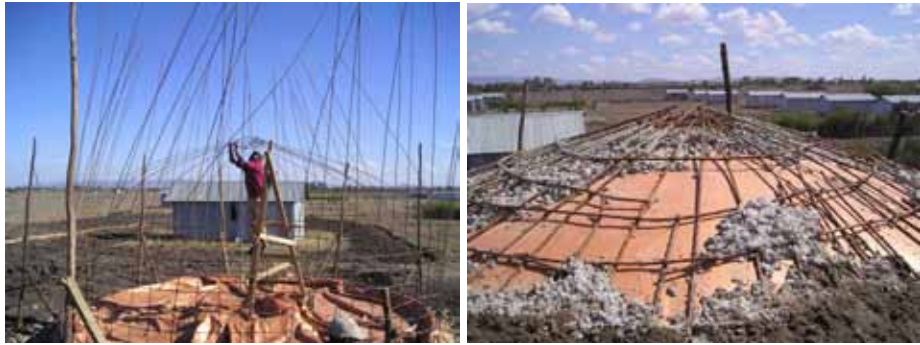
Figure 11.1: The airform did not reach the rebar cage in Ruia, Kenia [Spit]
